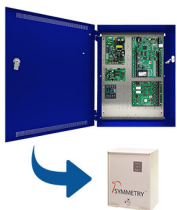
Replaced 30 AMAG proprietary panels with BluBOX Open Platform
